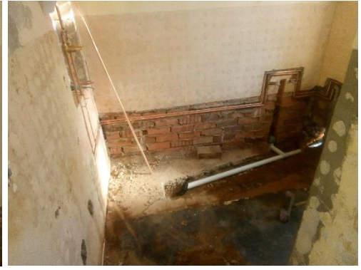
6 Shower drainage & wash basin plumbing
